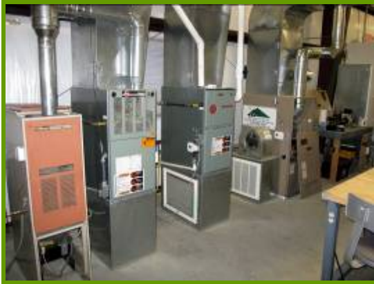
NRCERT Heating System Lab
