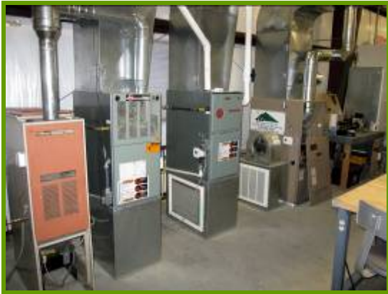
NRCERT Heating System Lab
