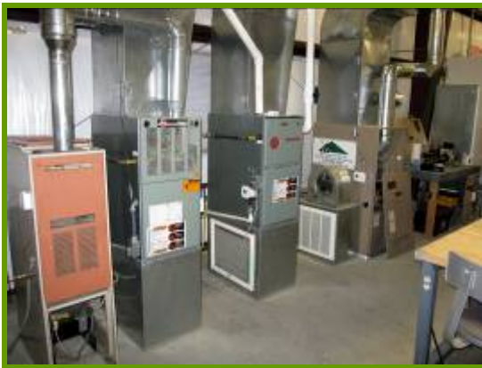
NRCERT Heating System Lab
