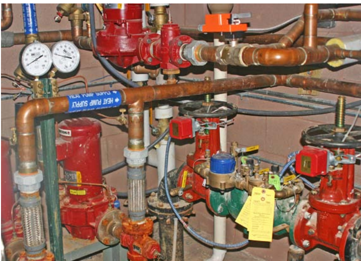
FIGURE 7. Geothermal HVAC system pipes and pumps (with valves to fire sprinkler system).
